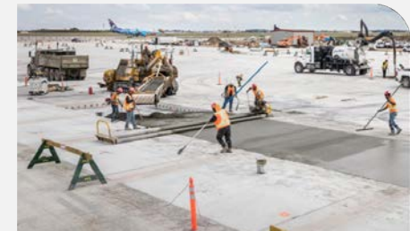
Calgary, AB – East Deicing Apron Owner: YYC Calgary International Airport CO 2 Saved: 160 tonnes
